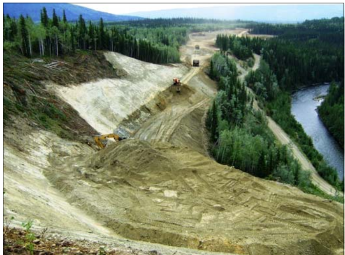
A closer view of the cleared penstock route and the location for the portal, which is the area where the penstock will enter underground.
