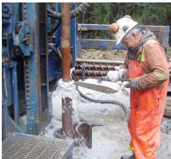
Bedrock drilling is necessary to help determine engineering design for Mayo B.
