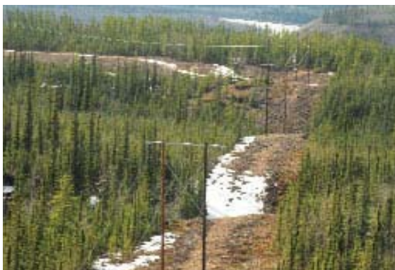
A section of the first phase of the Carmacks-Stewart transmission line. Photo: Ron Threkeld
