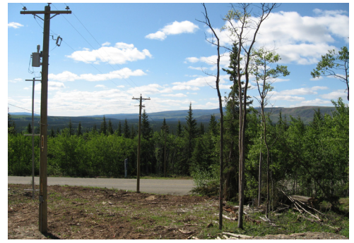
Distribution line from the Stewart Crossing substation to the community
