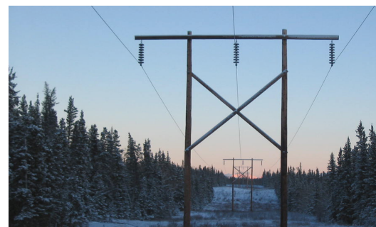
A 138 kV H-Frame Transmission Pole Whitehorse-Aishihik-Faro Transmission Line
