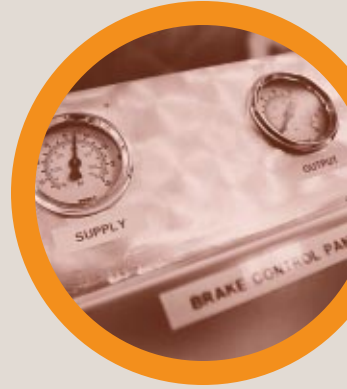
A SECTION OF A CONTROL PANEL AT YUKON ENERGY'S MAYO FACILITY
