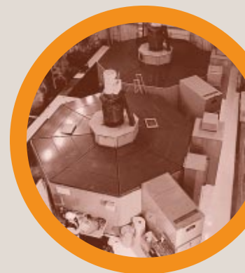
AISHIHIK HYDRO TURBINES
