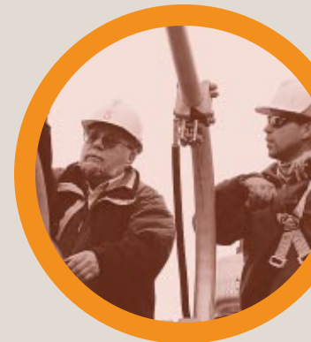
SUBSTATION ELECTRICIAN ED CHAPLIN (LEFT) AND MAINTENANCE ELECTRICIAN NICK BALDERAS (RIGHT) MAKE REPAIRS TO A SUBSTATION
