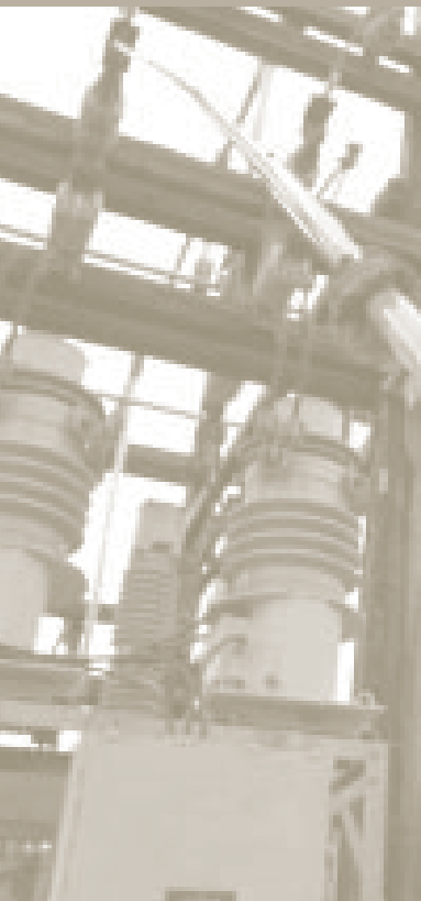
Yukon Energy employee Nick Balderas works at one of the company's sub-stations – Derek Crowe
