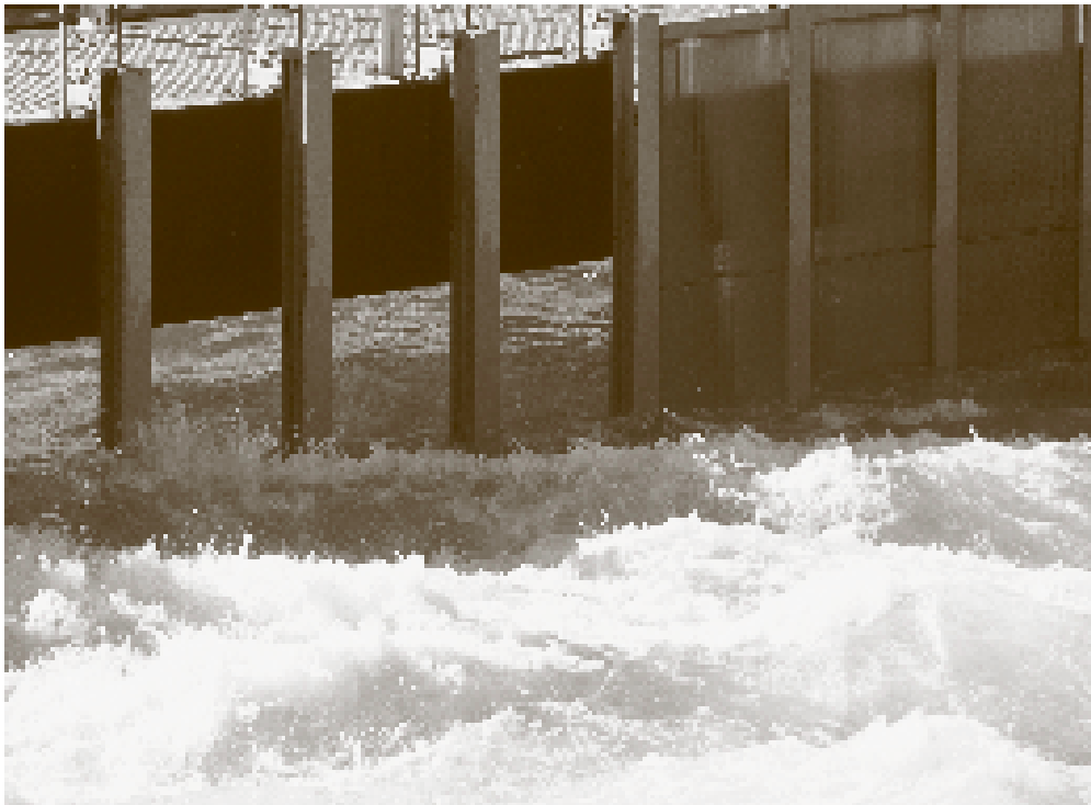
Missing fish screens from the Yukon River near the Whitehorse facility. The screens were carried into river as a result of the high water and heavy current. – Archbould Photography
