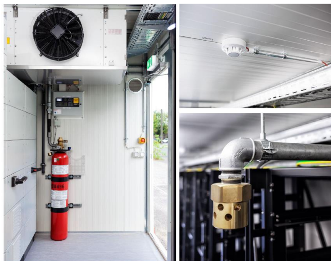
Figure 4-5: Sample of fire protection system, showing pressurized container of fire suppressant on left side, the fire/smoke detector in the container on the upper right, and the nozzle for dispensing the fire suppressant if required, on the bottom right.
