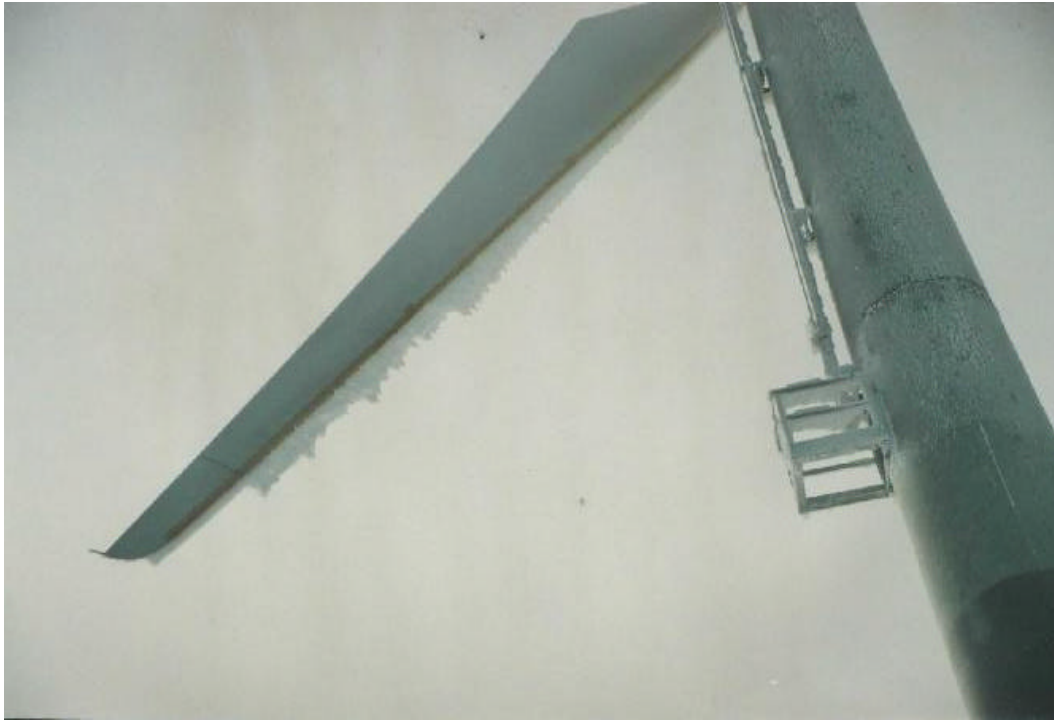
Photograph 5: wedge shape build up from back, note clear back of blade – leading edge heaters not working
