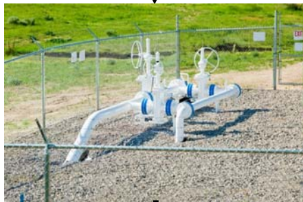
Natural Gas Transmission Pipeline
