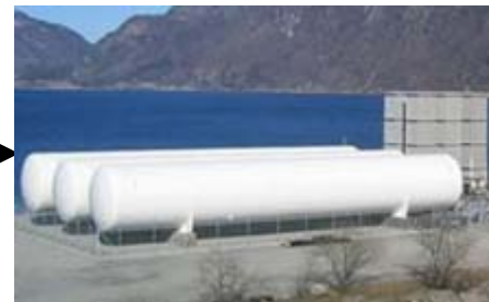
LNG Receiving, Storage and Vaporization
